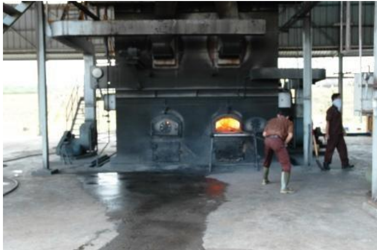
Lampiran 5 - Keadaan Boiler PT SBPU
